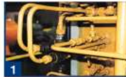
place of installation
