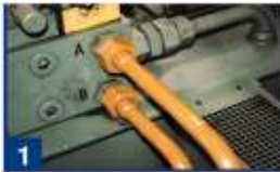
place of installation
